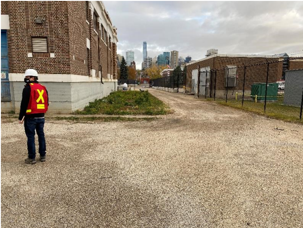
Above: Water ponding in drive lane east of the Switch House
