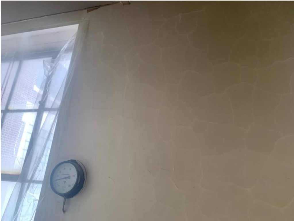
Above: Switch House – Drywall damage on 2 nd floor
