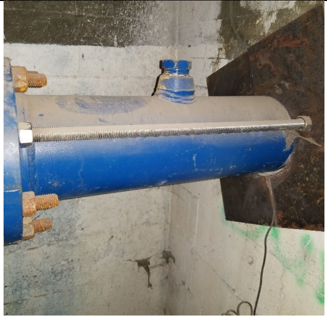
Above: 100mm domestic water connection North
