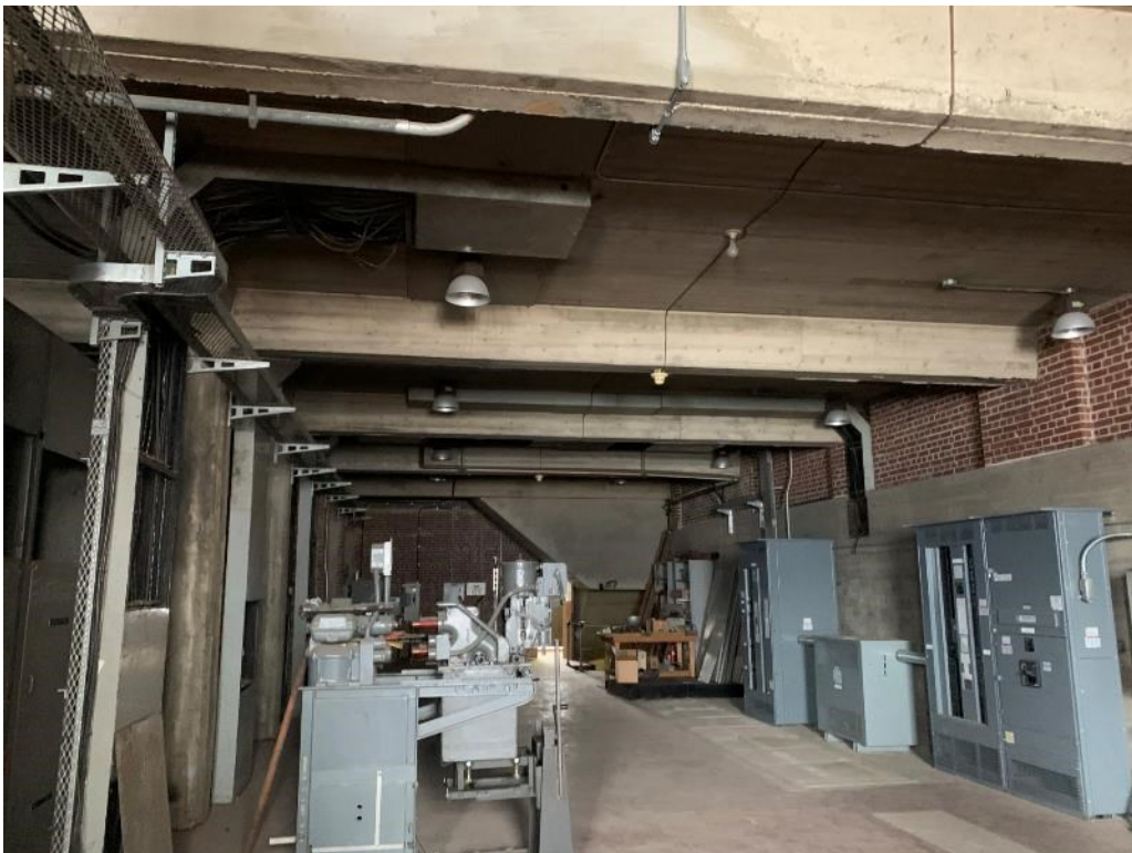
Above: Switch House – Main Floor
