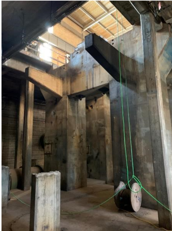
Above: Boiler Hall – Basement Pedestals
