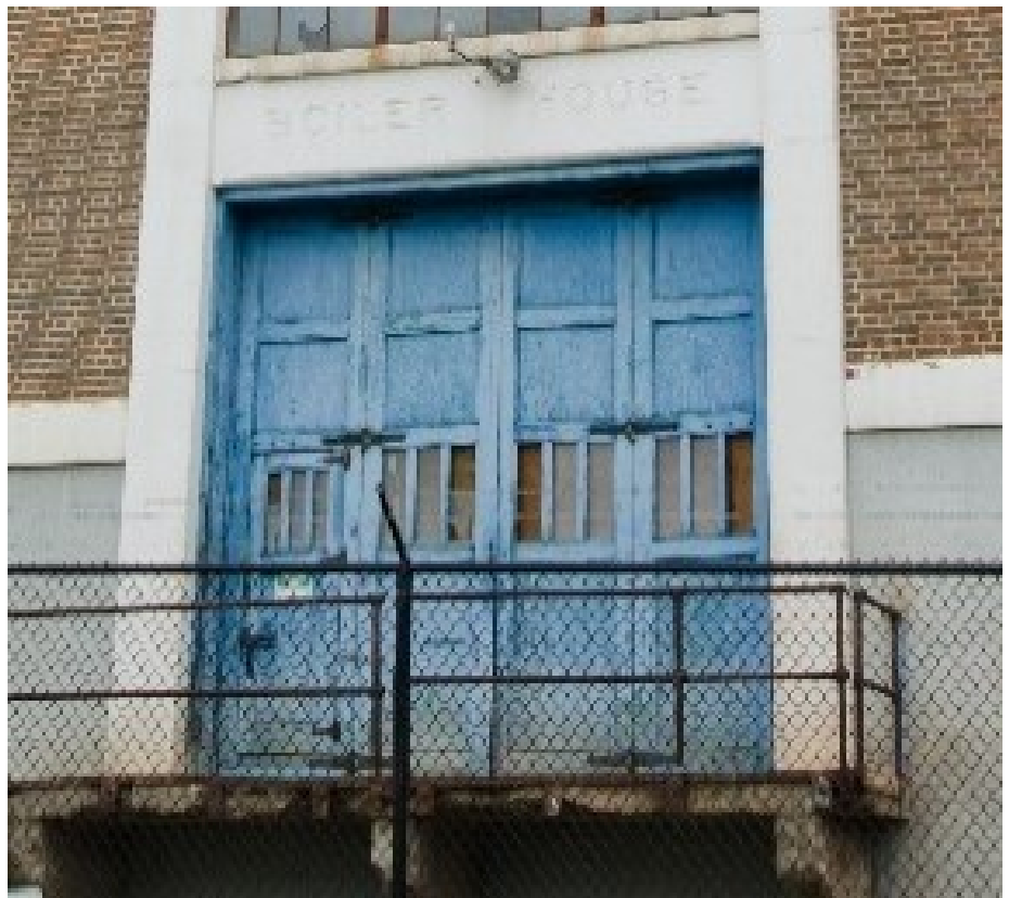
D9 Quadruple Folding Panelled and Glazed Door, West Elevation: Paint is failing and wood is deteriorating as expected with deferred maintenance over time. Some glass lights are broken or missing. Conservation is necessary.
