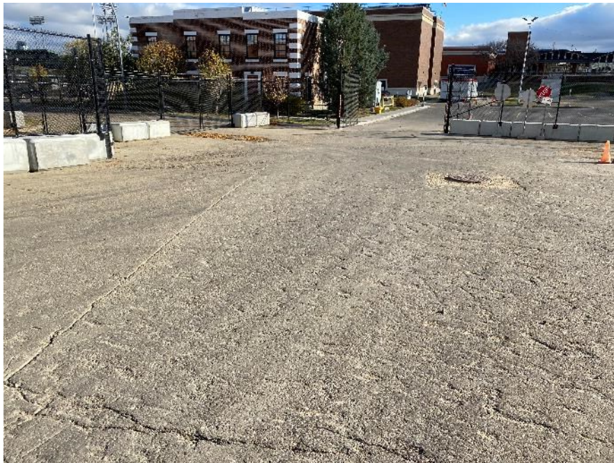
Above: Damaged asphalt from heavy equipment
