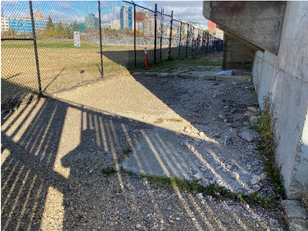
Above: Exterior concrete landing and curb deterioration
