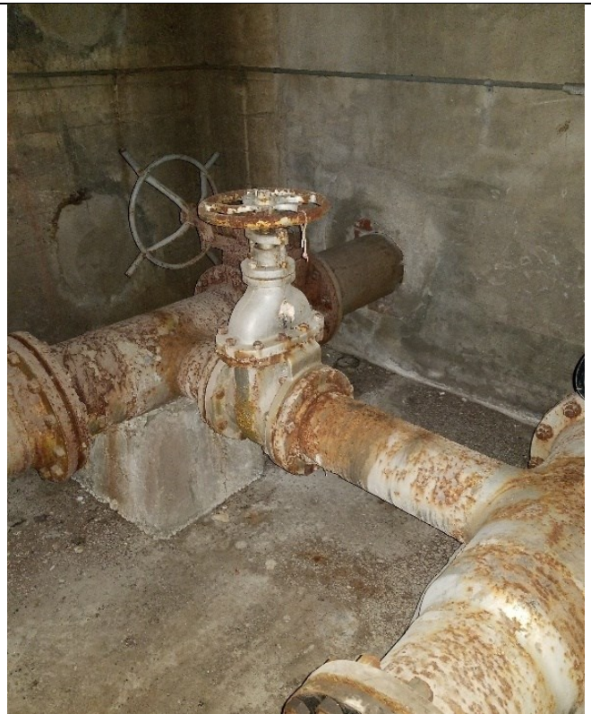
Above: 300mm steel gas piping
