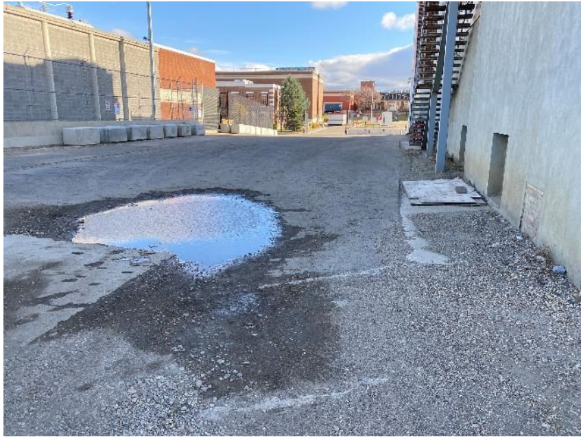
Above: Water pooling in settled asphalt area north of the Low Pressure Plant
