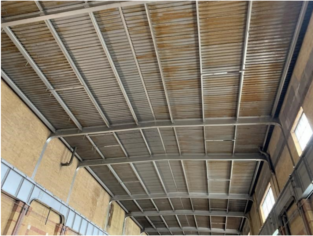
Photo 1: Turbine – Roof Structure – Rusting of Deck
