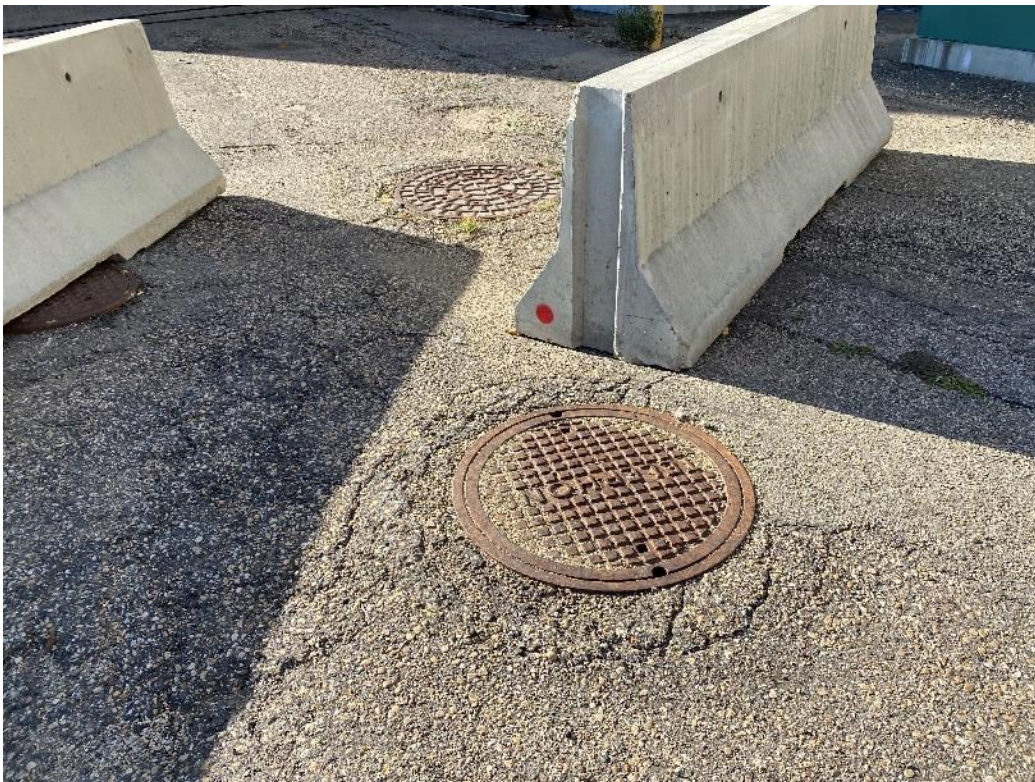
Above: Settlement and cracking around Manholes and vaults
