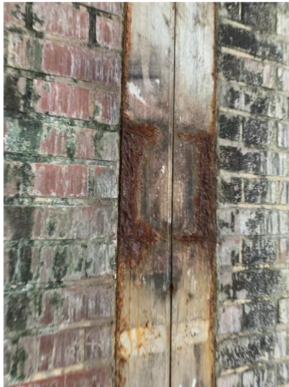
Above: Boiler/Turbine Hall – Column Rust on shared Wall
