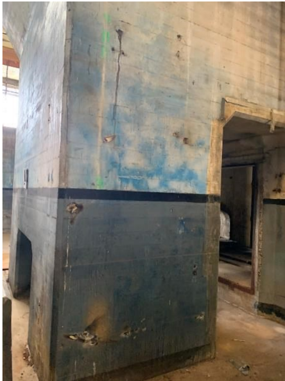
Above: Turbine - Basement Pedestal
