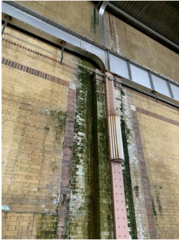
Above: Turbine –Column with Organic Growth
