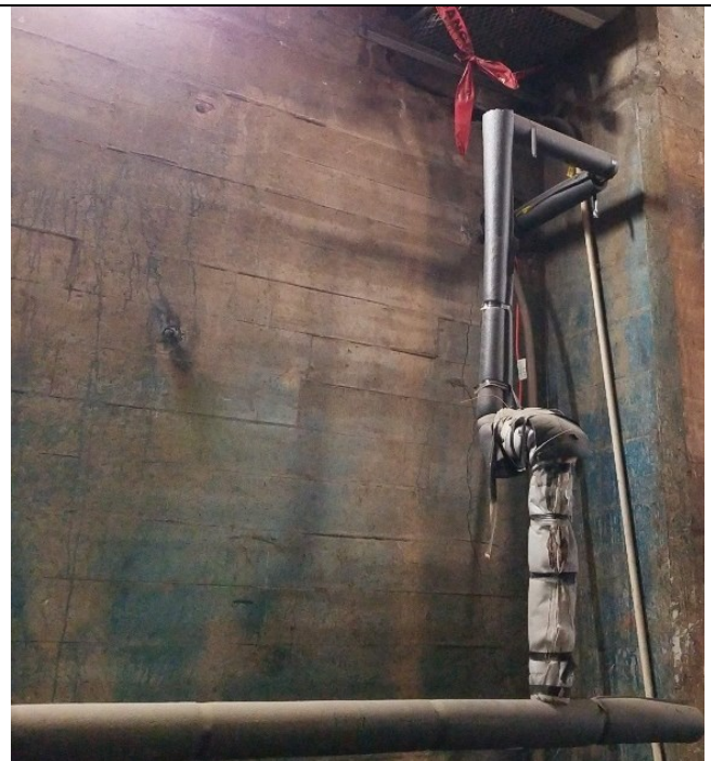
Above: 150mm domestic water connection from EPCOR Treatment plant
