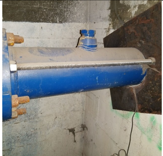
Above: 100mm domestic water connection North
