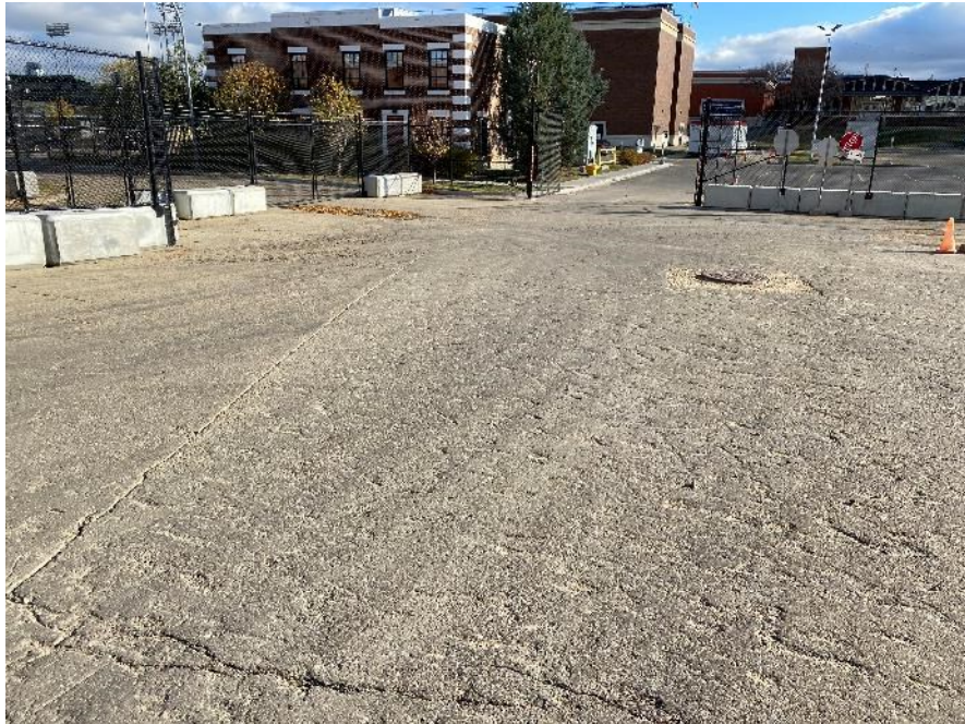
Above: Damaged asphalt from heavy equipment
