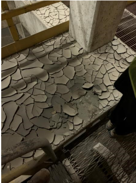
Above: PH2 – Lower Level Structures (Sediment on Structure)
