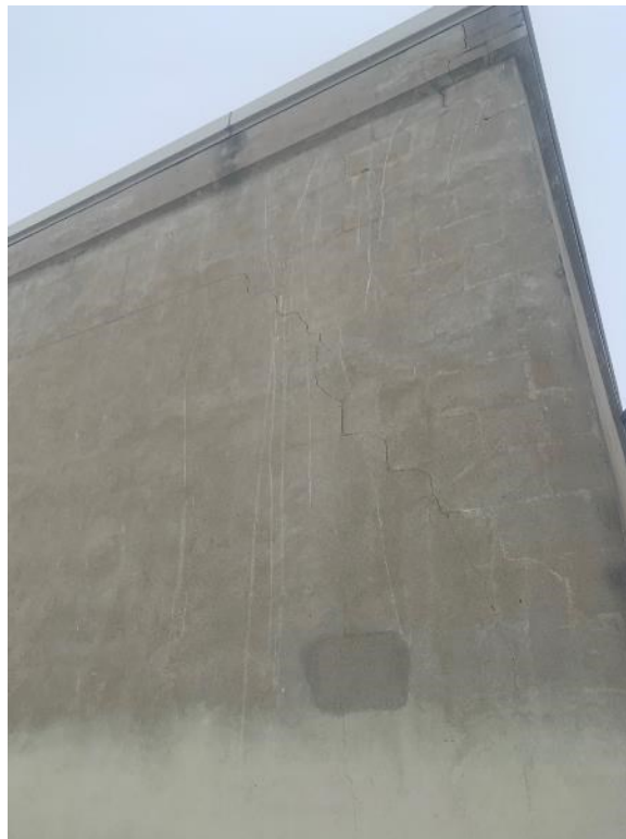
Above: PH2 - Exterior Cracking
