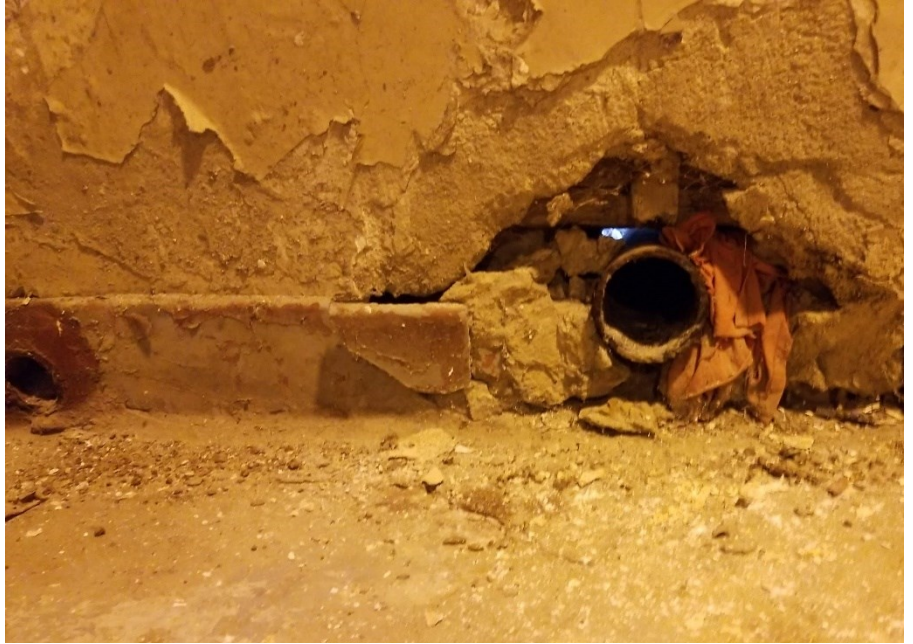
Above: Abandoned piping penetration
