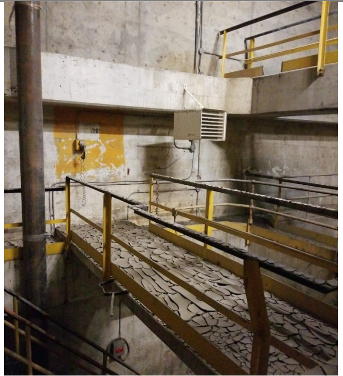
Above: Sediment deposits at the highwater mark
