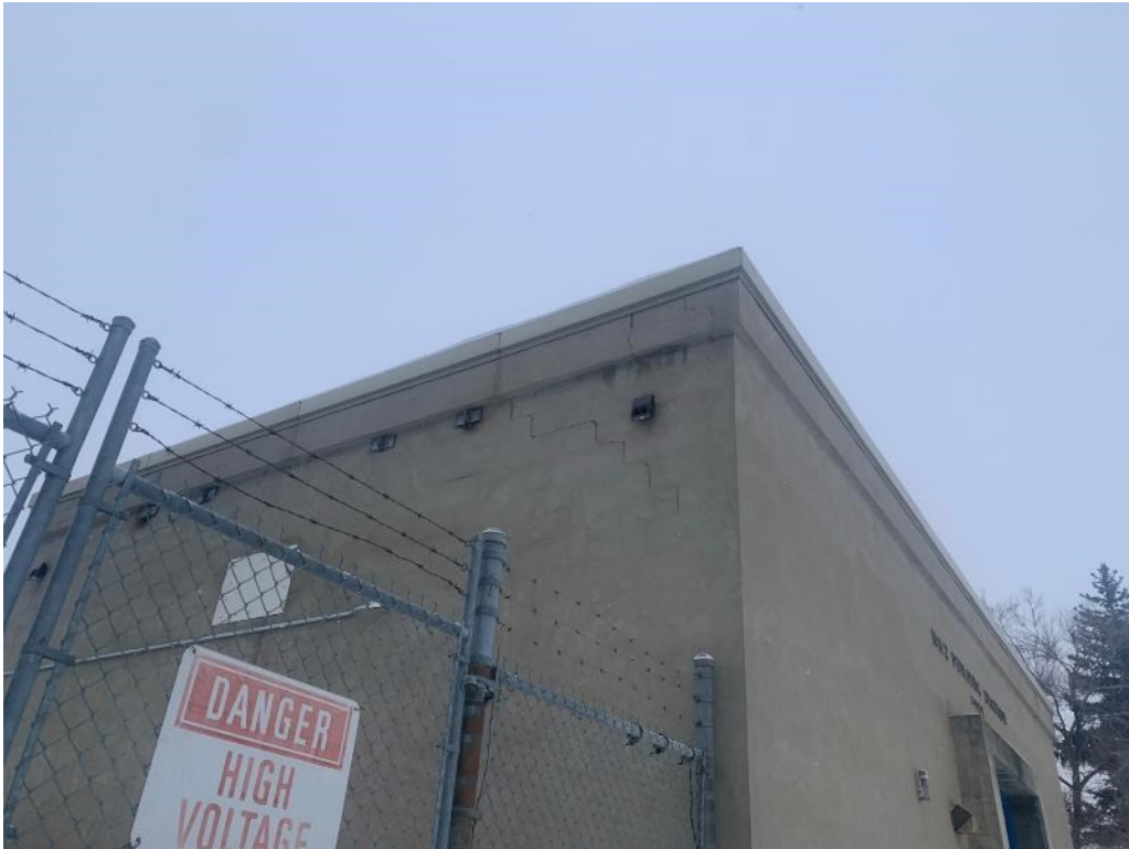
Above: PH2 – Exterior Cracking
