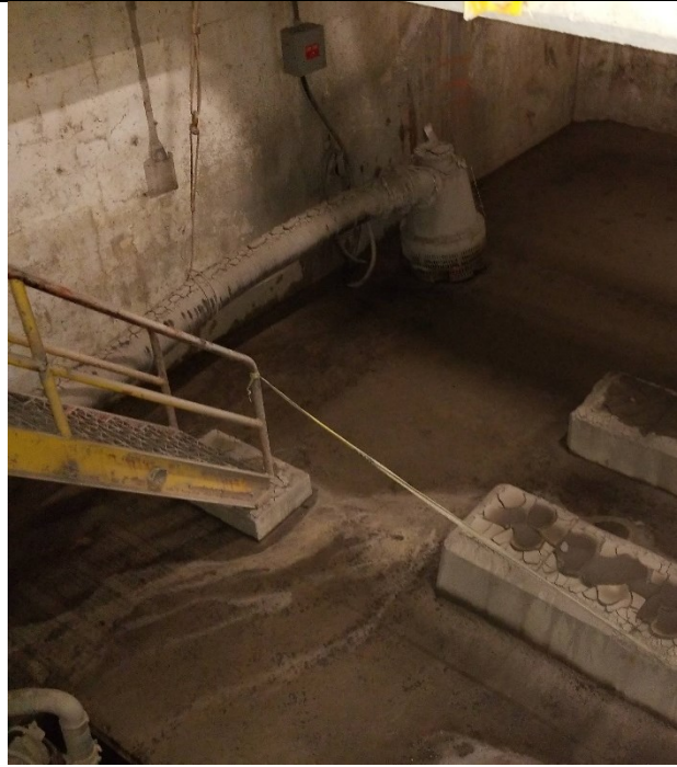
Above: Basement level dewatering pump
