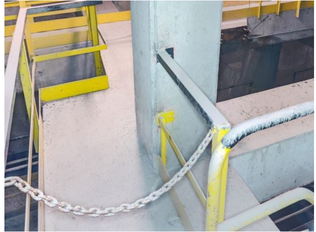
L4: Thicker Sediment Deposits
