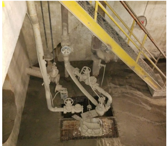
Above: Basement level sump and pump
