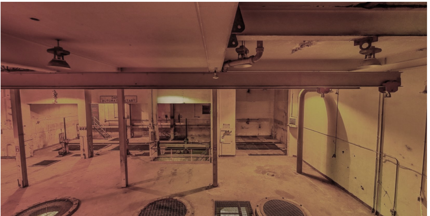
Figure 58: Pump House #2 main operating floor, Basement level 1. (Cloud360, 2020)
