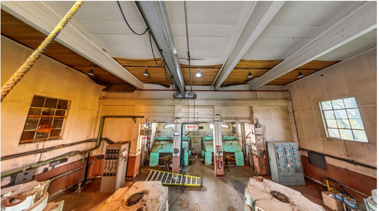
Figure 49: Pump House #1 Main/Operating Floor. (Source: Cloud360, 2020)
