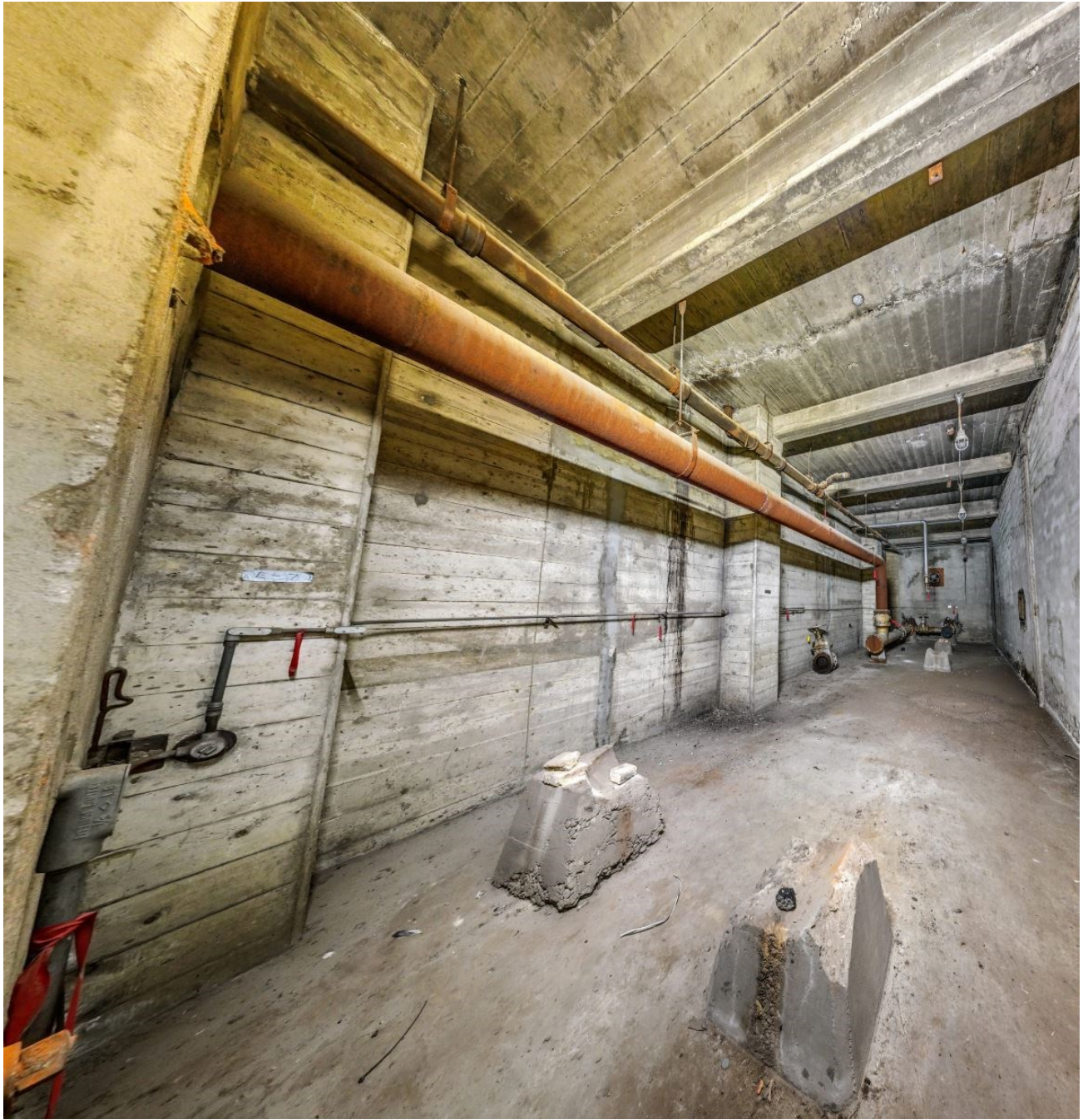
Figure 23: Natural Gas related pipes, dating from the era of boiler cessation of coal, 1940s-1950s. (Source: Cloud360, 2020)
