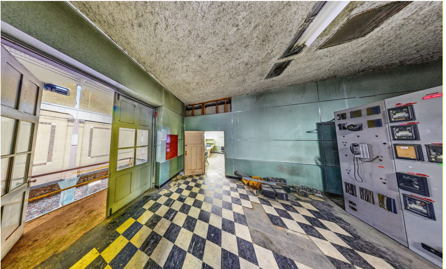
Figure 43: Switch House, Plant Control Room. (Cloud360, 2020)
