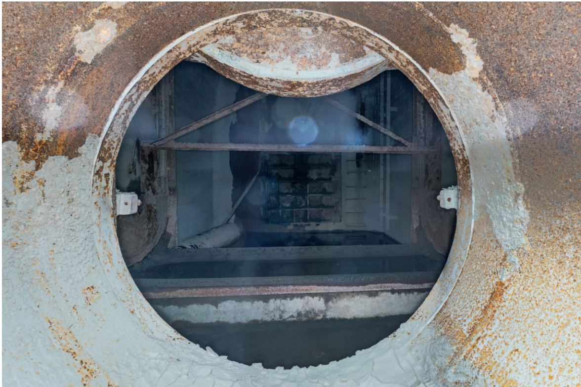
Figure 63: Wet Well Unit #4 (Cloud360, 2020)
