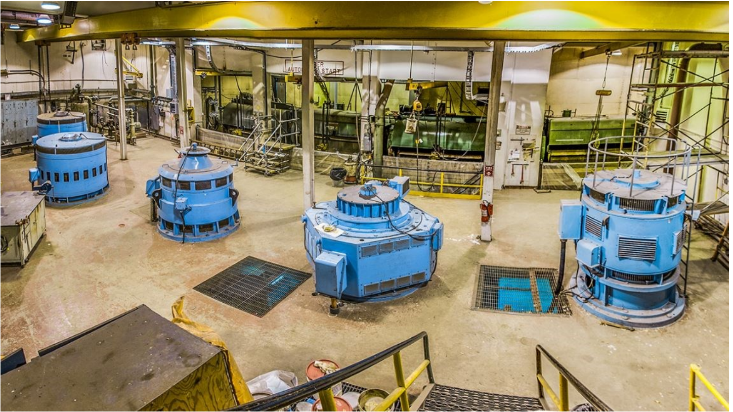
Figure 144: Operating floor of Pump House #2 while still in operation. Note the similarities in configuration with Pump House #1. Date Unknown. (Source: EPHF)
