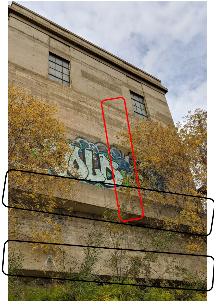
Figure 54: Red rectangle hi-lights the vertical crack in the centre of the south elevation of Pump House #1, and the later additions of the two horizontal ferro-concrete beams are encircled in black. (Source: Oxland, 2020)
