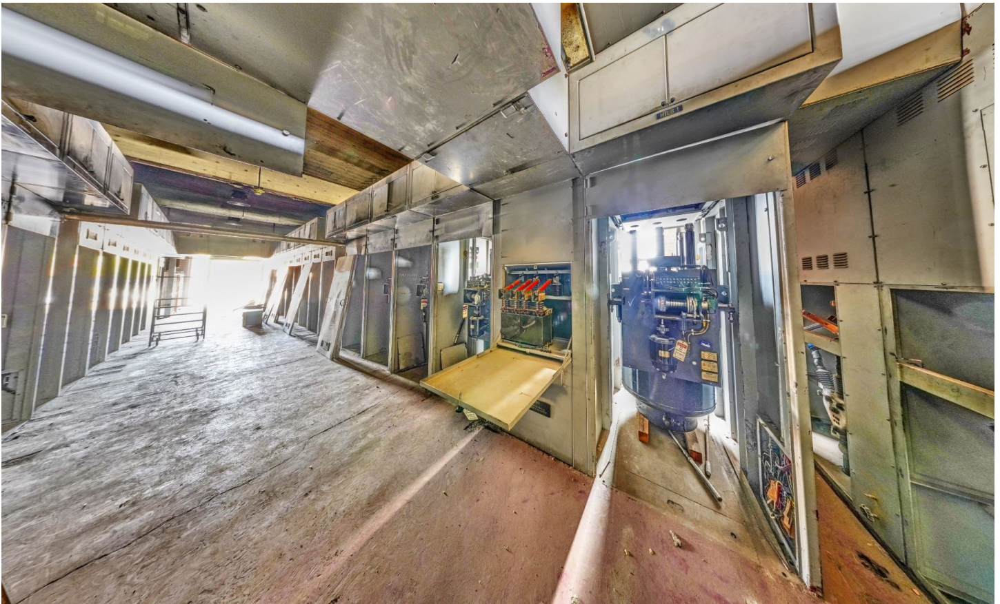
Figure 45: Large refrigerator sized breakers and drop down cabinets with transformers. (Source: Cloud360, 2020)
