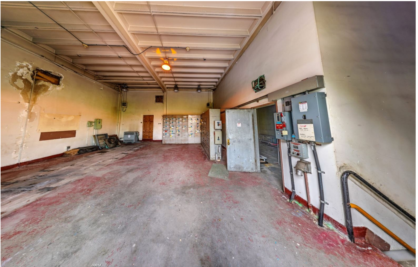
Figure 57: Pump House #2 main floor electrical rooms. (Cloud360, 2020)
