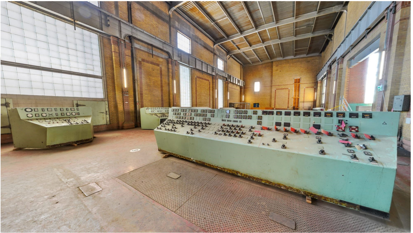
Figure 36: The Brown & Boveri control panel disassociated from the HPP associated control room, now in the Turbine Hall.
