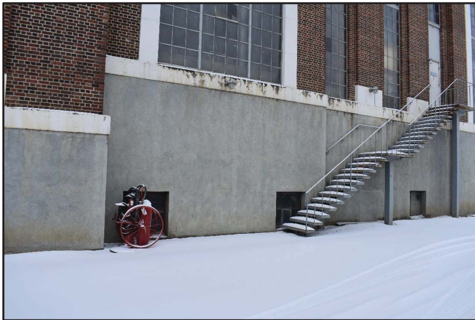
Figure 12-1: Example of Exit Discharge (Exit D4) Non-Compliant with Exit Exposure Concerns
