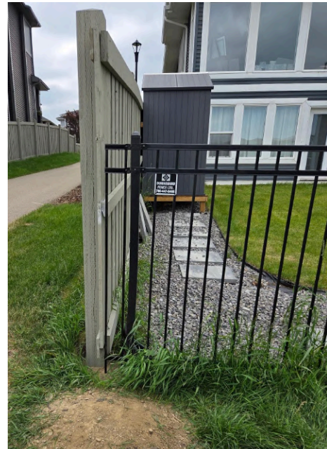
If the gap between 2 fence terminal posts exceeds 100 mm, a solution may be proposed by the Consultant/Contractor.
