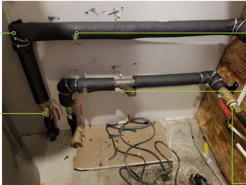
Image 2: Example of unacceptable insulation work
