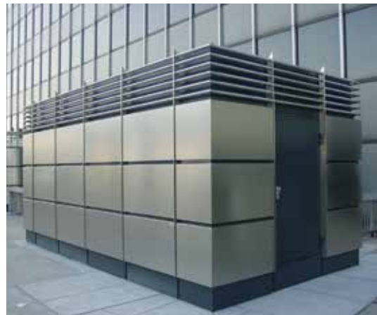
An at-grade utilities screen that is consistent with the architectural character of the principal building [13].
