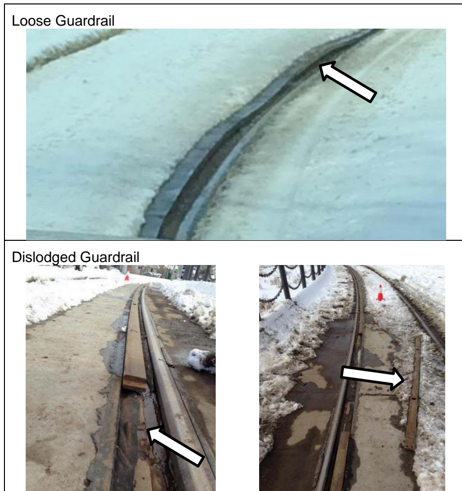
Figure 3 – Guardrail Track Issues
