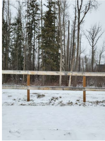
Post and Rail fencing require wood stain
