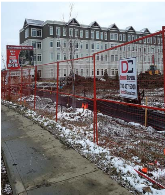
Construction fencing prohibits inspection of trees and turf
