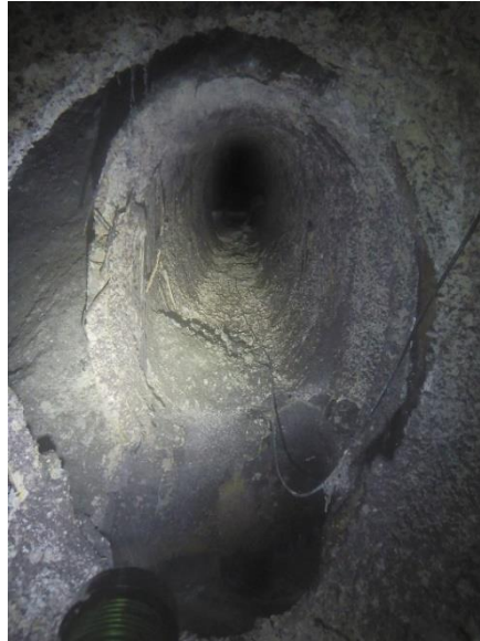
Figure 2.0-4 Large Void Upstream of Reach 49
