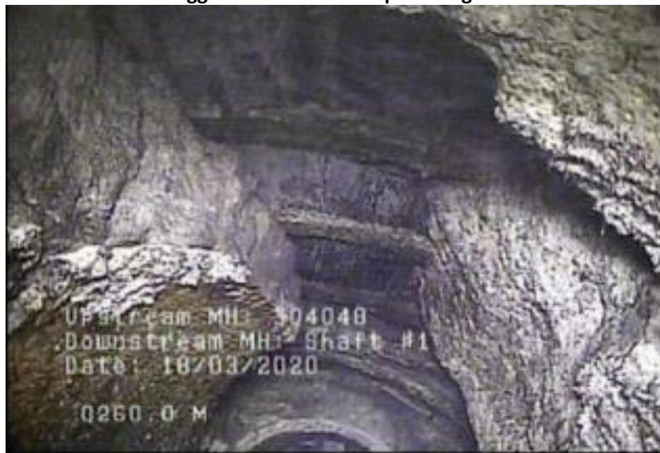
Figure 2.0-2 Duggan Tunnel - Close-up Missing Wall
