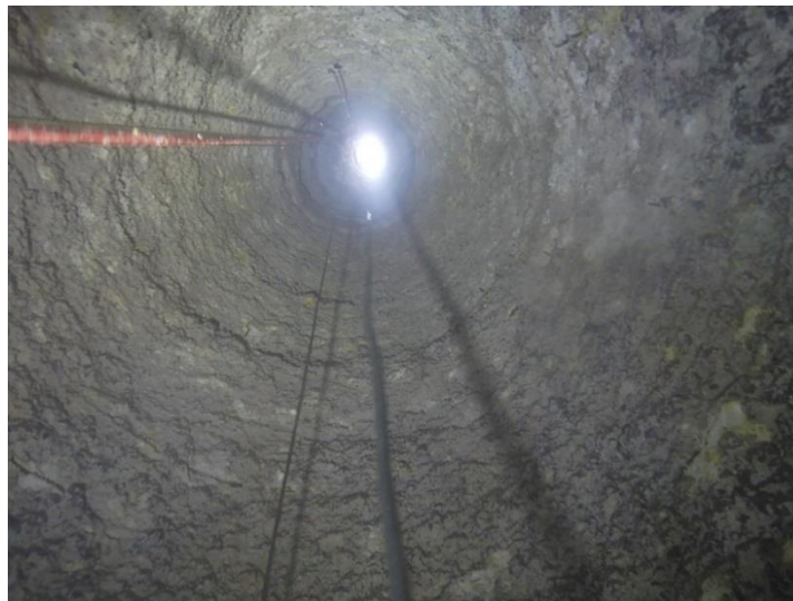
Figure 2.0-5 Severe Corrosion in Manhole 246631 At Junction of Reach 40 and 49
