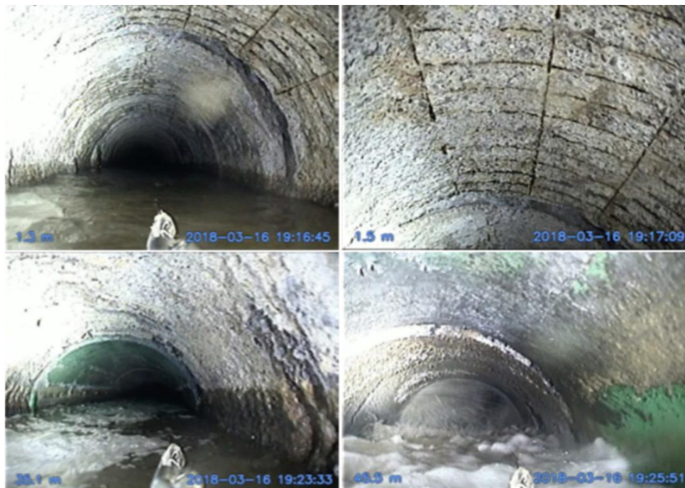
Figure 2.0-4 Deterioration of Small Trunks
