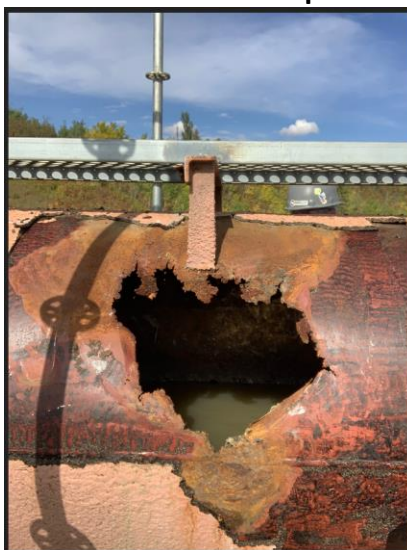
Figure 2.0-7 Failed Section from the Steel Pipe on the Trestle
