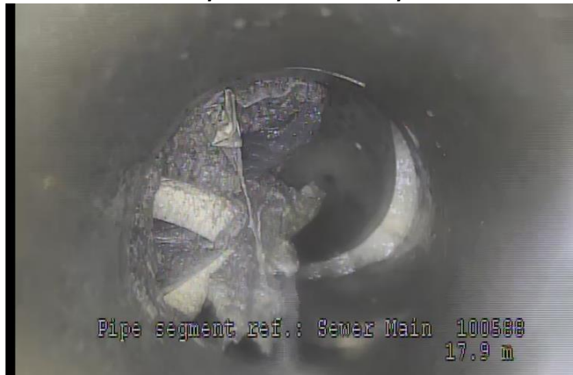
Figure 2.0-2 Broken Sanitary Service Line at Entry to Mainline
