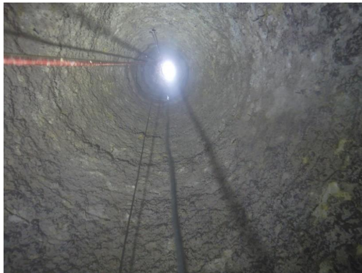
Figure 2.1-3 Severe Corrosion in Manhole 246631 and Junction of Reach 40 and 49
