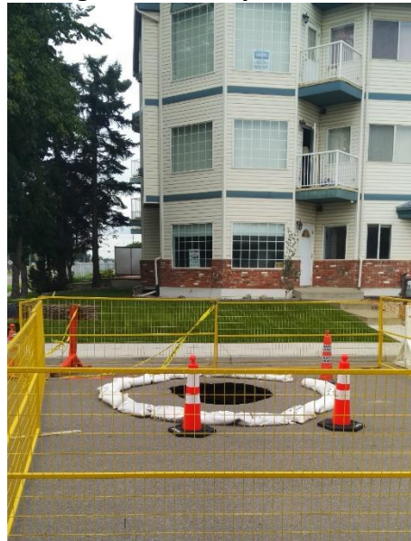
Figure 2.0-3 Image of Roadway Subsidence
