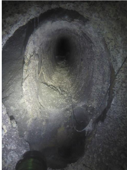
Figure 2.1-2 Large Void Upstream of Reach 49
