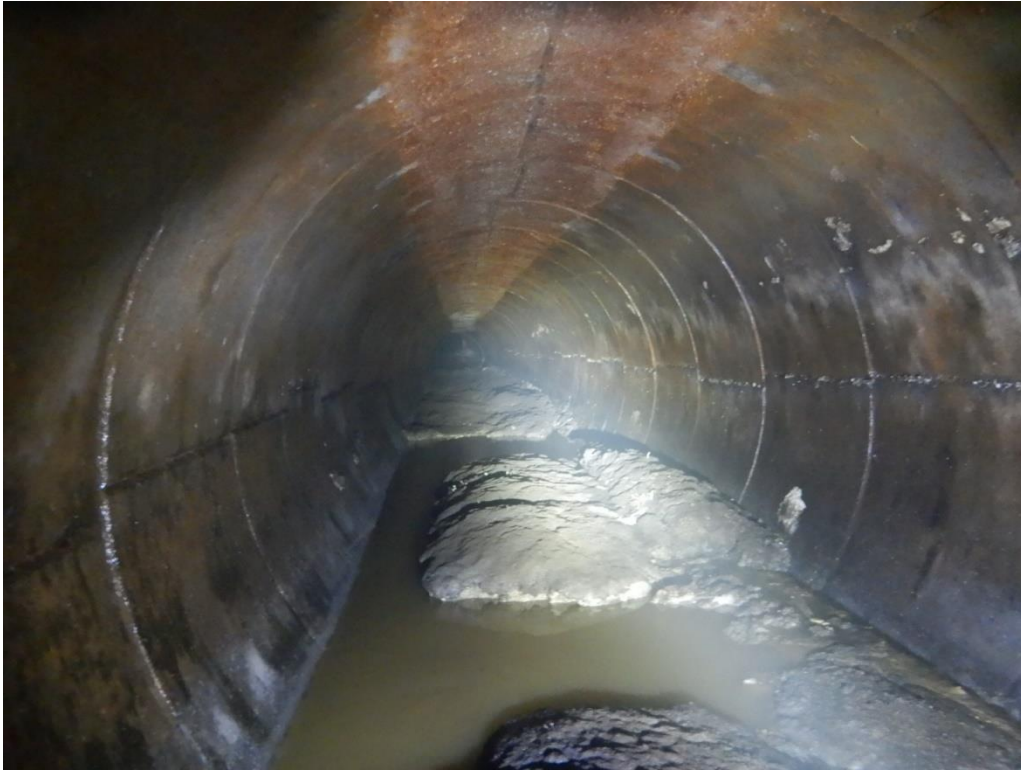
Figure 2.4.5-6 NL1 Tunnel solid accumulation
