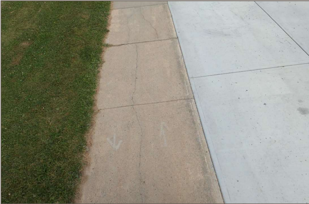
Photo 10: 178 Street, August 2020: Minor mortar flaking on concrete apron on right side of photo.
