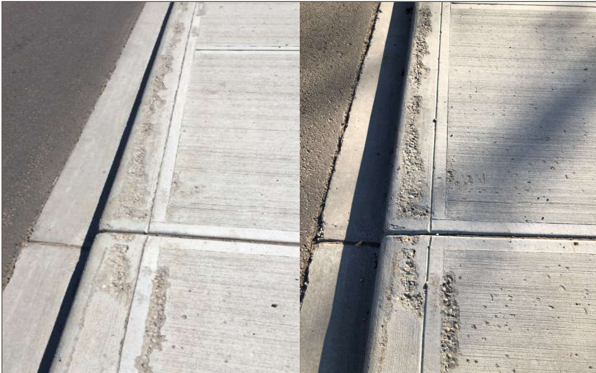
Photo 3: 111 Avenue: July 2019 photo on left, September 2020 photo on right. No noticeable difference in damage to volume of concrete removal by snow clearing equipment.
