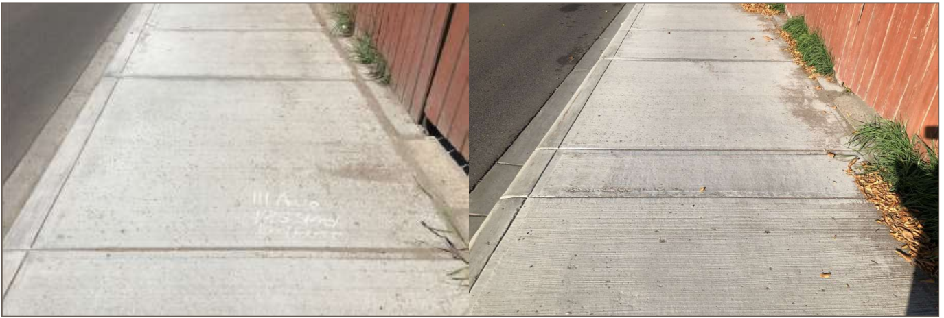
Photo 2: 111 Avenue: July 2019 photo on left, September 2020 photo on right. No noticeable change in mortar flaking volume.
