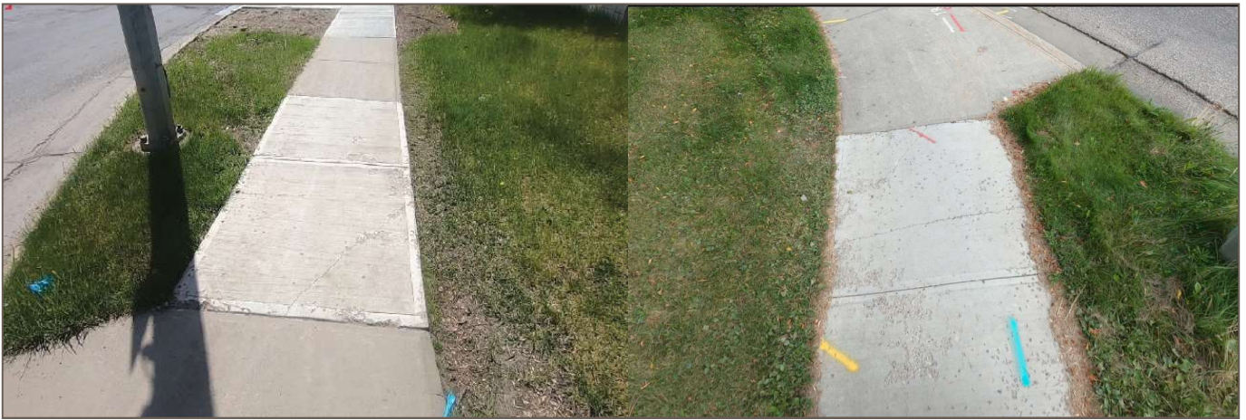
Photo 9: 178 Street: May 2019 photo on left, August 2020 photo on right. Severe scaling on panel likely construction related. Likely to be removed.
