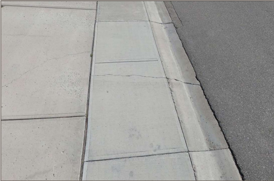
Photo 14: Laurel, August 2020: Random cracking in sidewalk panel.
