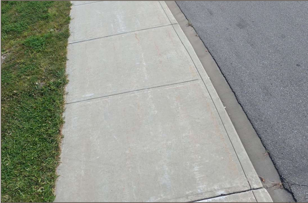
Photo 16: Laurel, August 2020: Scraping on sidewalk caused by snow removal.
