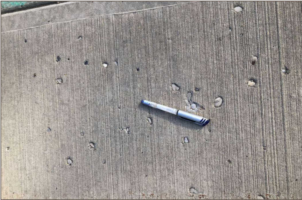
Photo 1: 122 Street near Fox Drive, September 2020: Mortar flaking on sidewalk surface caused by drying of surface above coarse aggregate.
