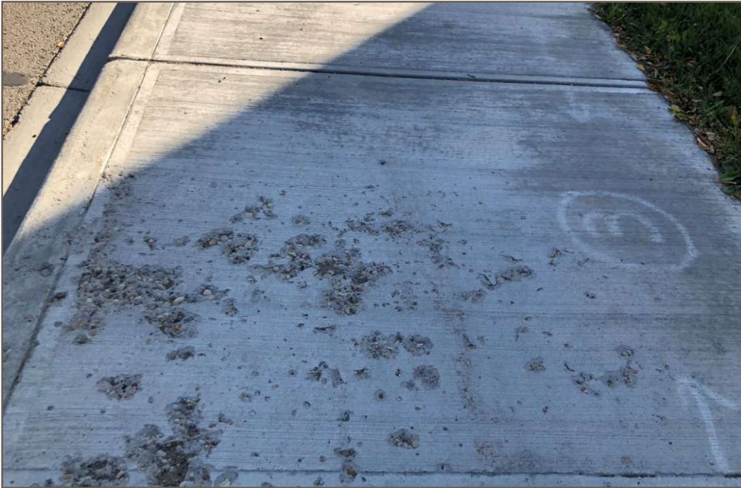
Photo 6: 111 Avenue, September 2020: One panel with severe scaling, likely to be removed.
