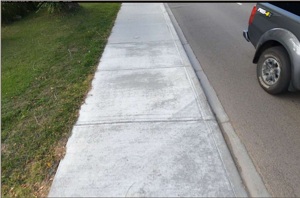
Photo 4: 111 Avenue, August 2020: Difference in concrete surface colour due to removal of curing compound.
