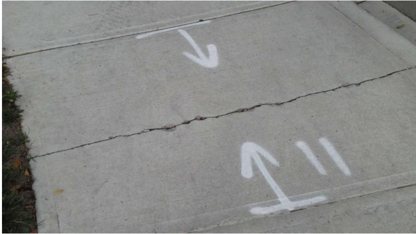
Figure 3 - Example of concrete deficiency marked for removing and replacement
