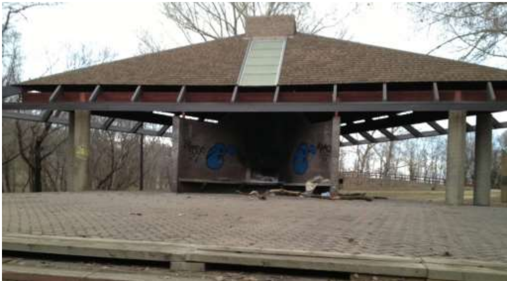
Plate 5.8. The picnic shelter and hard surface appear to be in disrepair and public fireplaces installed as part of the picnic shelter structure have been boarded over (April 2013).
